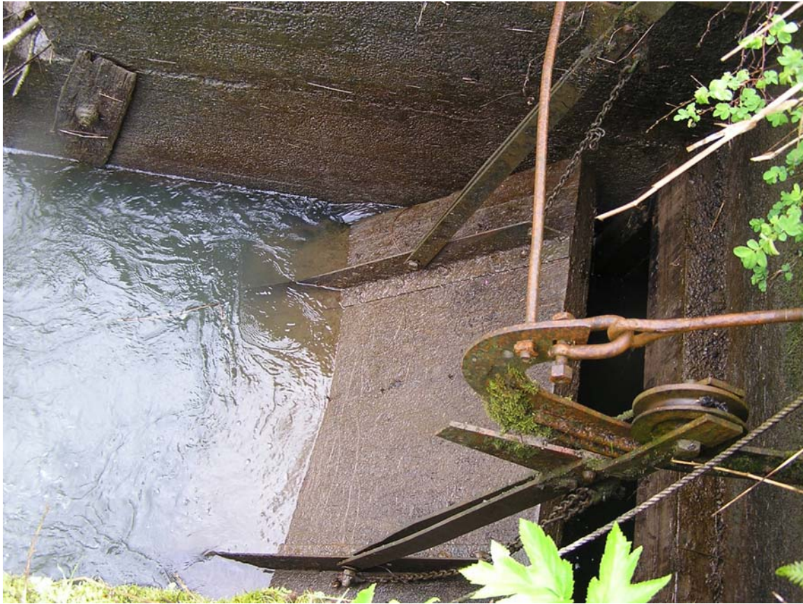
Figure 6. Damaged Tide Gate at W259+50 Slough (looking down, gate is wedged open)
