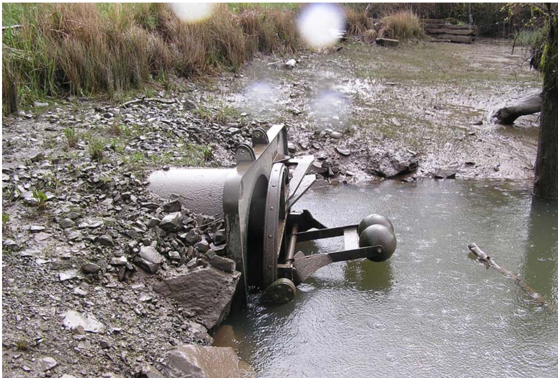
Figure 8. Partially Closed Tide Gate at W201+30 Slough
